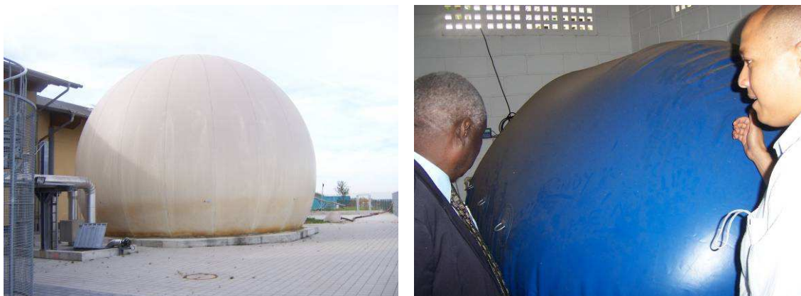
Figure 7.26 External low pressure gas storage tanks (RUTZ 2007)
