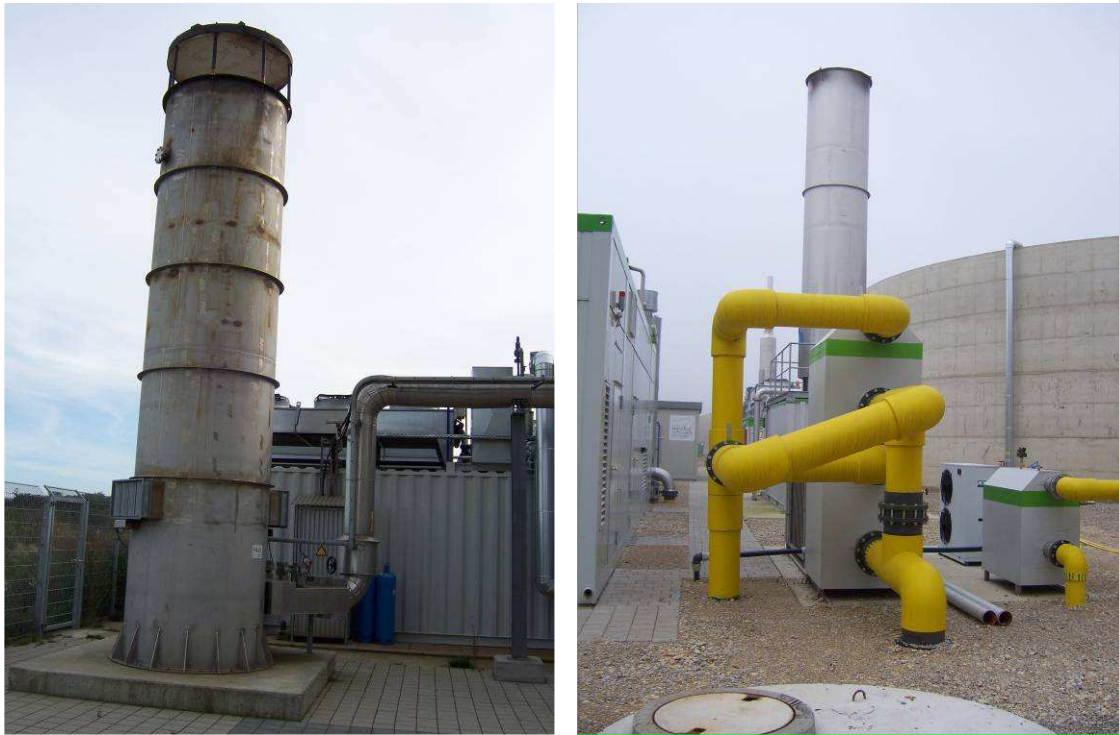
Figure 7.28 Modern biogas flares (RUTZ 2007)
