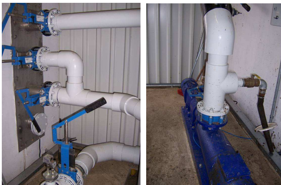
Figure 7.8 Stop-valves (left) and pumping system (right) (RUTZ 2006)
